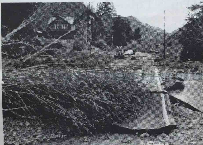
ROAD DAMAGE - Miami-Foley Rd damage near Shiffman Rd. (Nadine J. Calkins photo)
