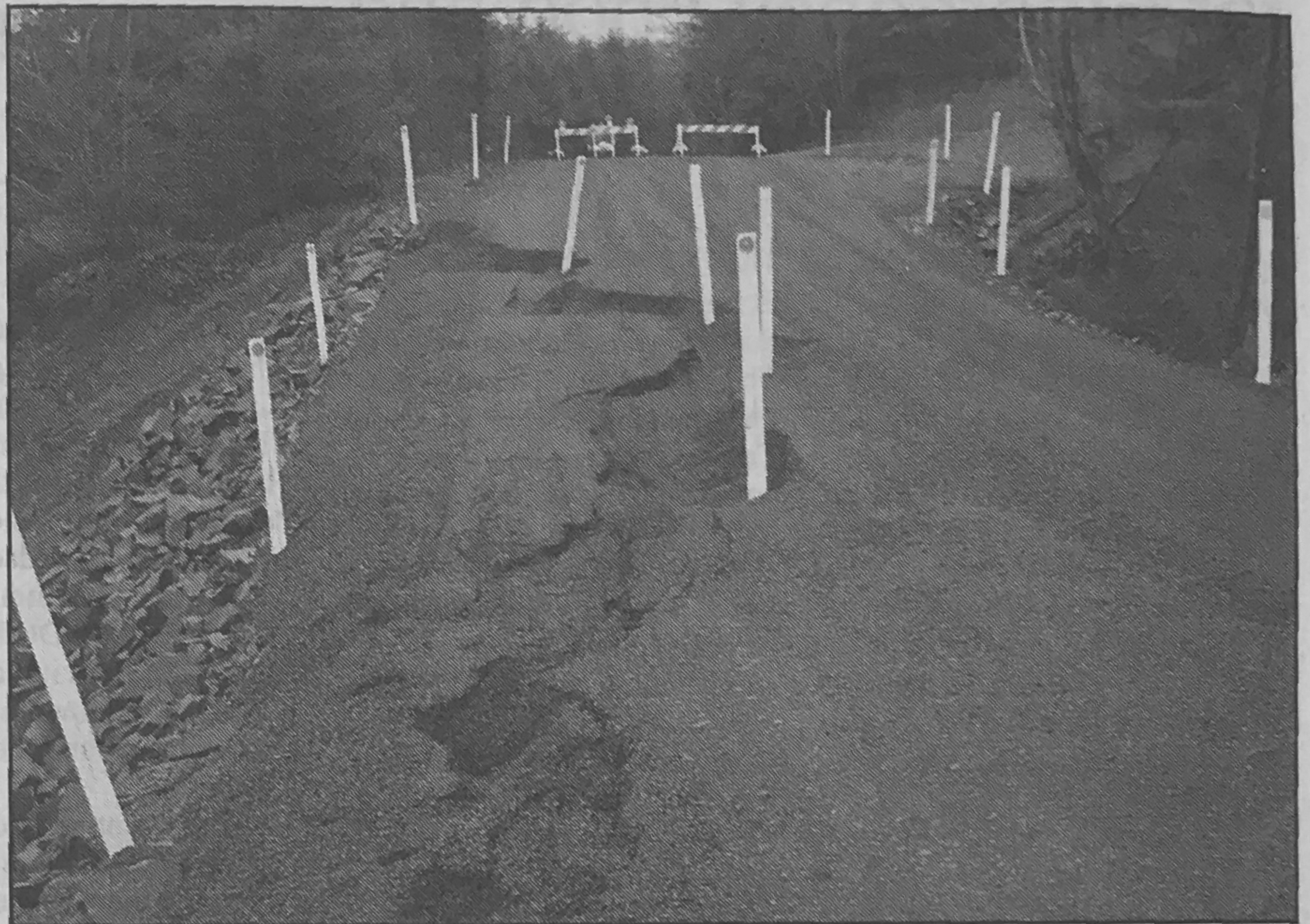
ABOVE: The Cape Meares Loop Road is closed 1.3 miles south of Cape Meares Lake due to a slide that took out the south bound lane. The road links the community of Cape Meares with Oceanside and Netarts. Cape Meares State Scenic Viewpoint is accessible north from Oceanside. The road will remain closed until further notice.
