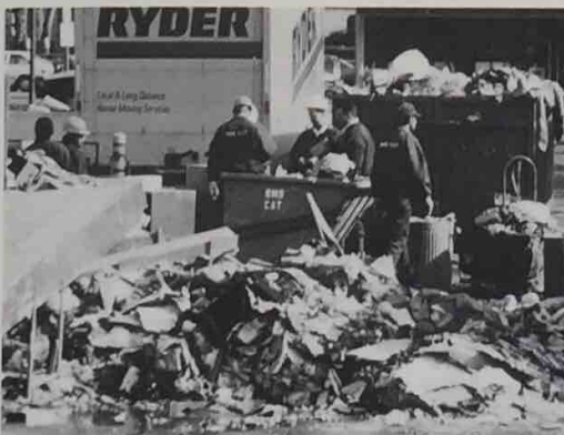
Forty-five large dumpsters were required to haul away the damaged remains of the building, totaling over 2.2 million pounds of garbage material.
